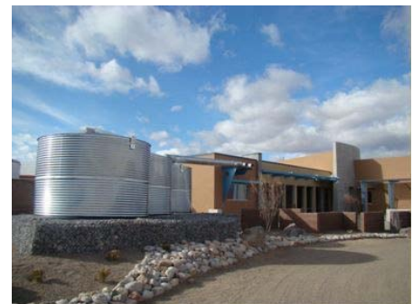
Rainwater harvesting with three above-ground cisterns providing 15,000 gallons of landscape irrigation water from 4,000 square foot roof area (Albuquerque, NM).
